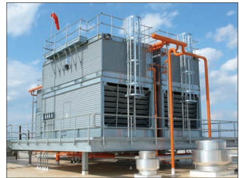
Multi-Cell CXVT Installation Showing Simplified Piping
